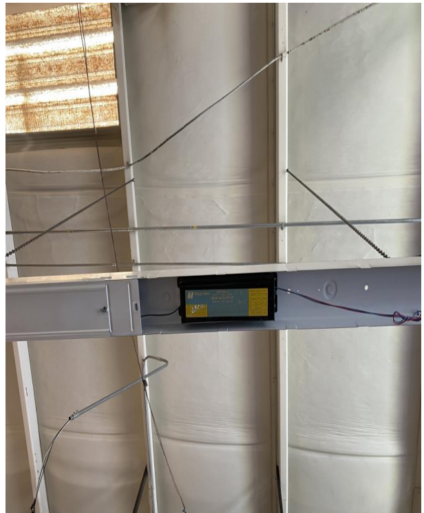
Photo 16 Comments: Non-PCB containing light ballast
