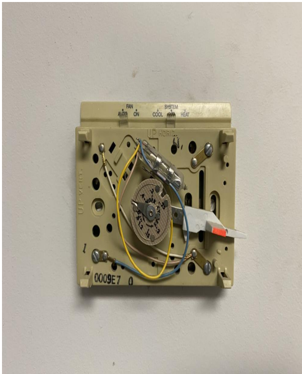
Photo 15 Comments: Mercury Containing Thermostat
