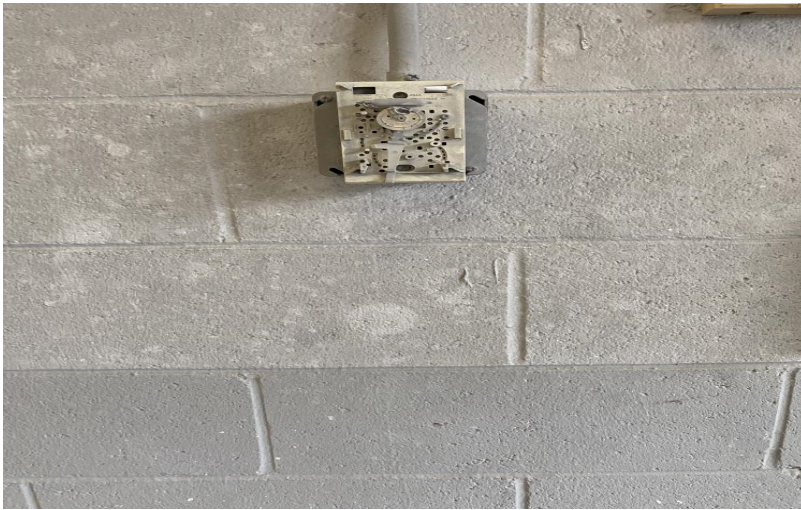
Photo 17 Comments: Mercury-containing thermostat
