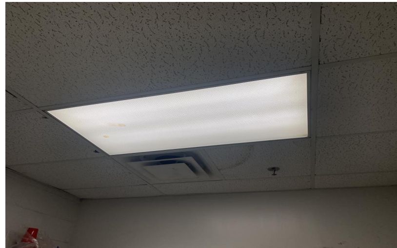
Photo 16 Comments: Break room light fixture
