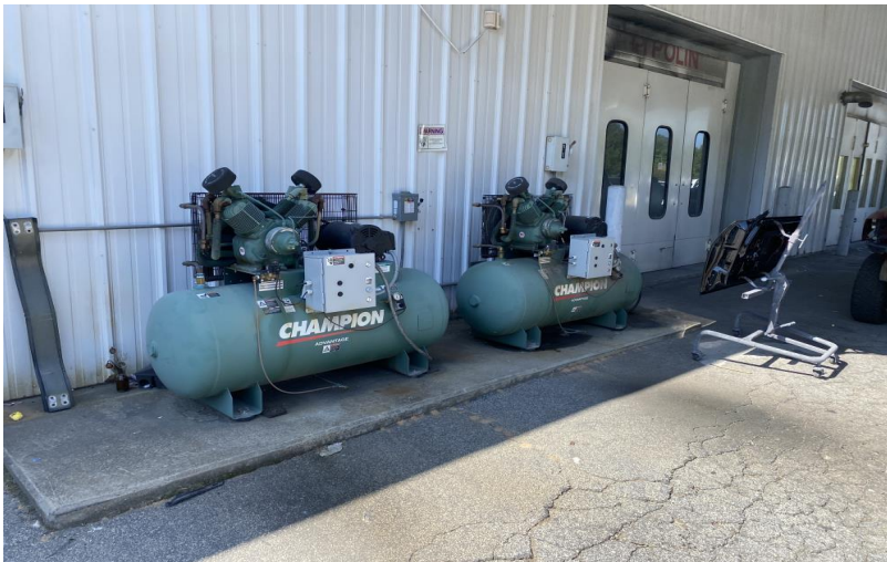
Photo 27 Comments: Air Compressors
