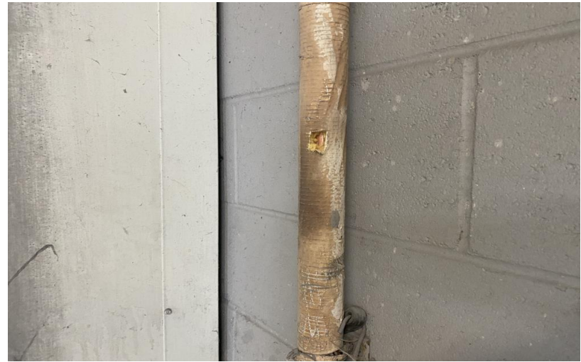
Photo 10 Comments: Pipe insulation
