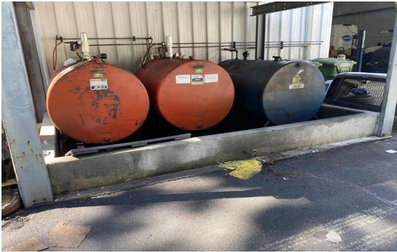
Photo 13 Comments: Used oil tanks on north exterior
