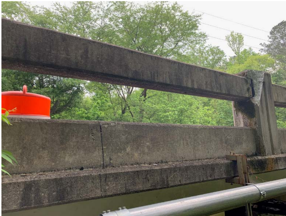
Honey Creek Road Bridge Rail Damage – picked up by GDOT Bridge program
